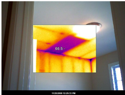
Purple area shows missing insulation in bedroom ceiling
