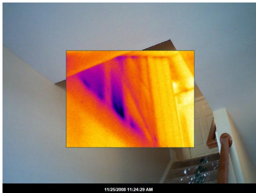
Purple area shows inadequate insulation at 3 rd floor stair
