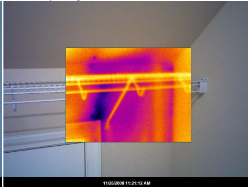
Purple area is inadequate insulation near knee-wall door
