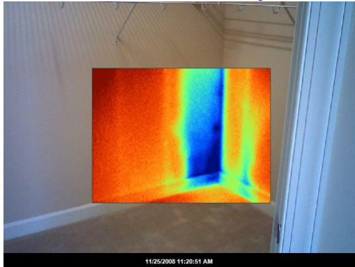
Blue area shows missing insulation in closet
